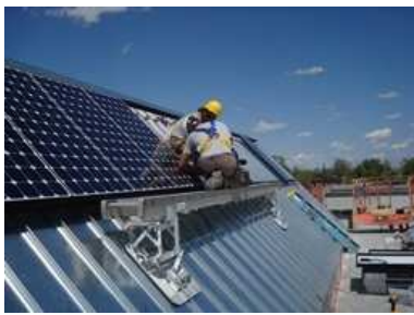
Photo: Independent Power Systems
